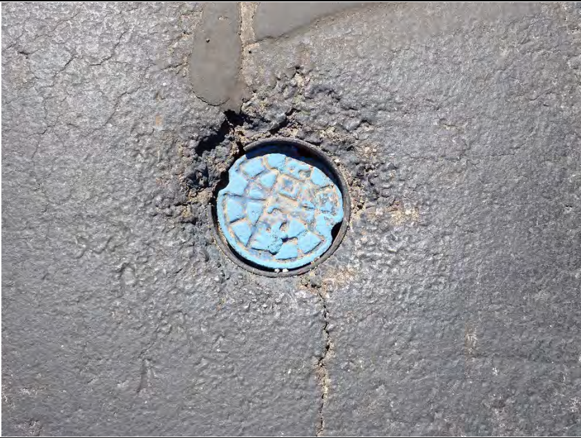
Typical piezometer protective casing and lid along dam crest.
