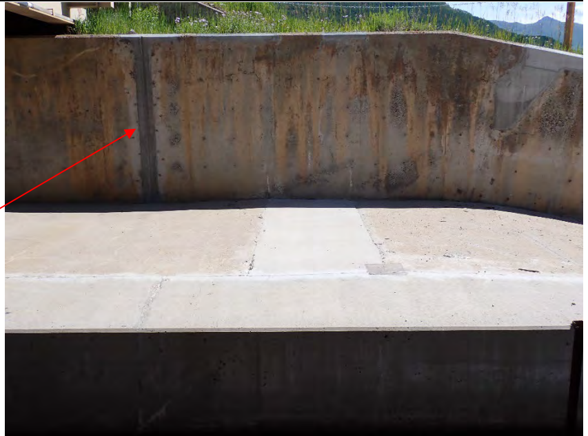
Left spillway wall with example of typical vertical crack repair and grouting.
