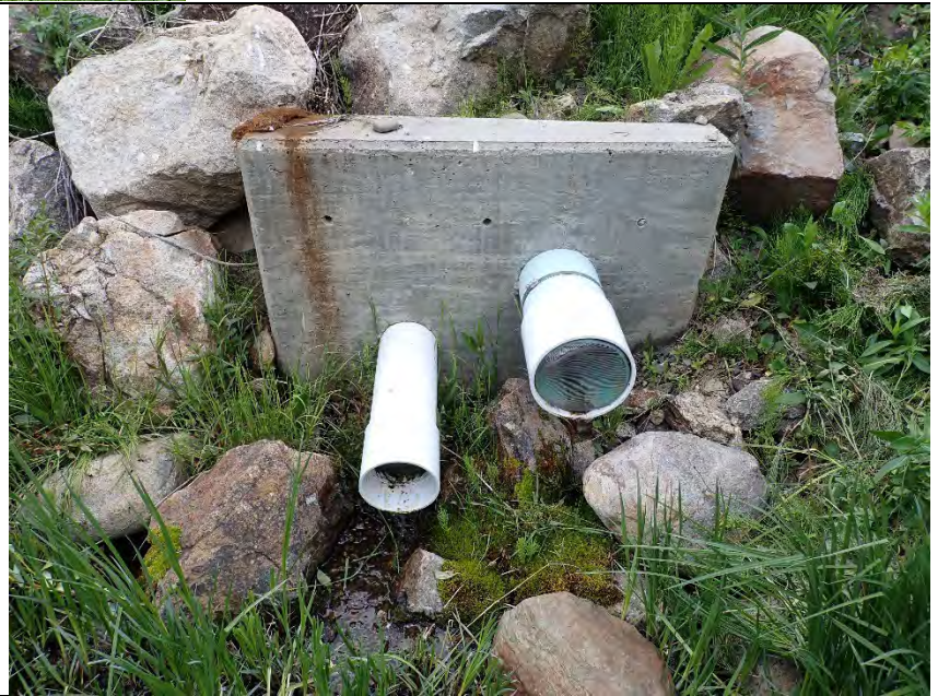
8-inch toe drain outfall (right in photo) 6-inch left abutment trench drain (left in photo). (Note: There is a possible discrepancy between C-1464C, Sht 5 and what is shown in this photo; sizes are swapped?)
