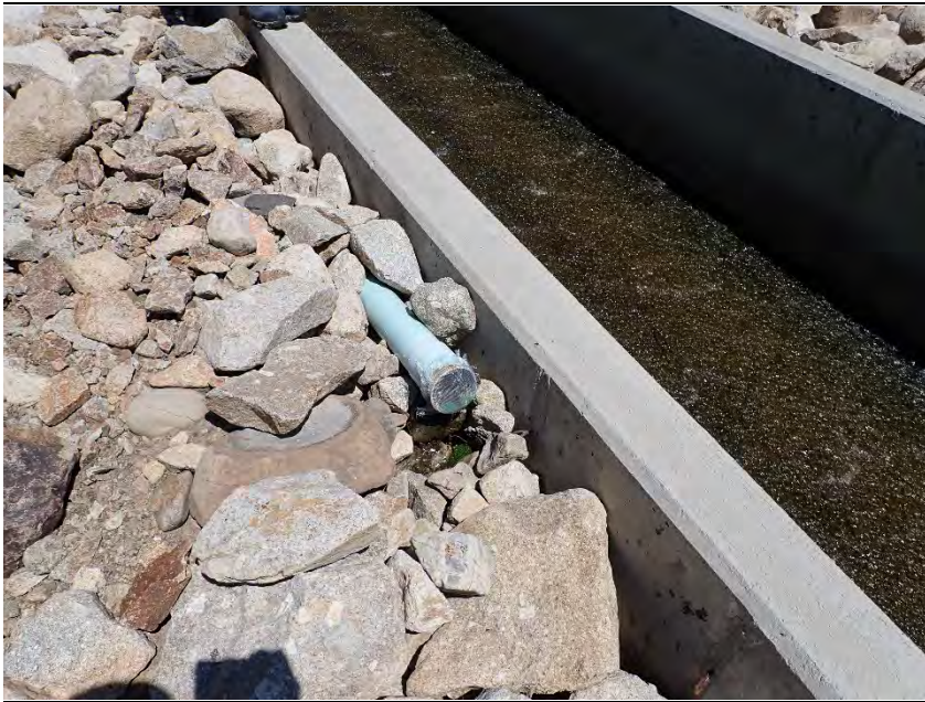
Typical low flow channel transverse joint drain outfall (right side shown).
