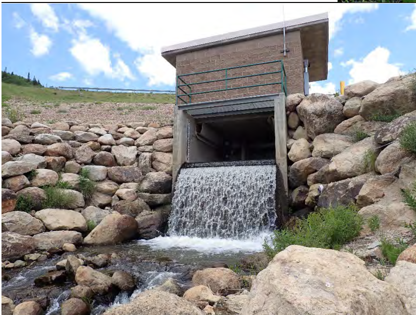
Outlet structure/pump station.
