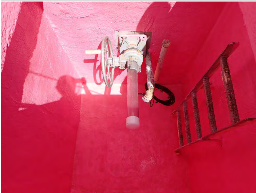
Internal view of outlet gate operator vault with recent (2023?) pink sealant coating.
