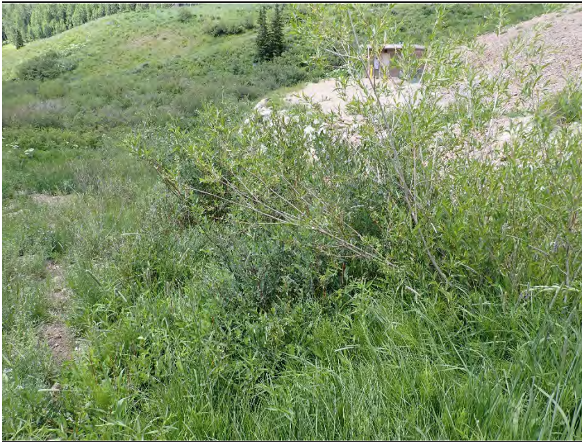
View looking downstream along contact groin of dam and left abutment. Willows partially obstruct access and visual inspection.
